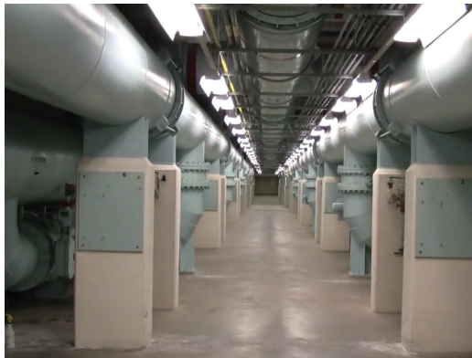
Filter plant pipe gallery
