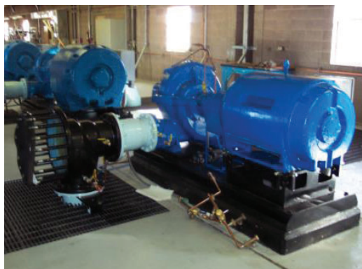
La Vista pump station
