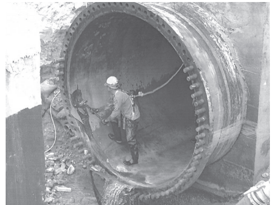
Water pipeline from Pueblo Reservoir
